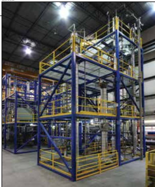
FIGURE 5. This image shows a modular cellulose-ethanol demonstration plant
