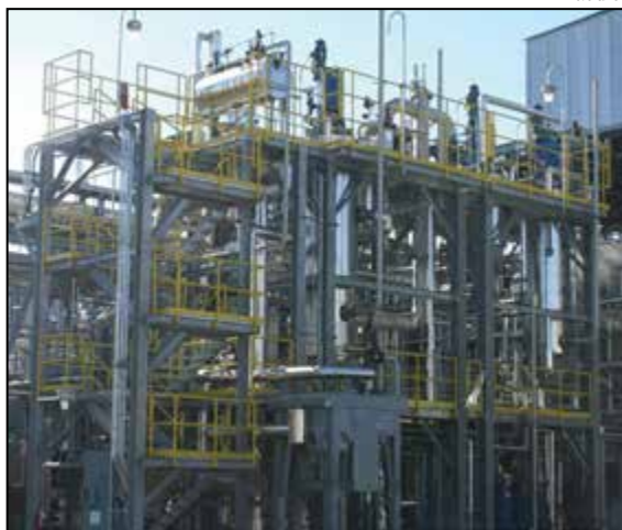
FIGURE 2. Shop construction is far more efficient than field construction and is not affected by weather or other plant-site activities. Thus, the modular process-system-design approach lowers overall project costs and shortens project schedules. Modular project execution greatly reduces site construction work and its associated plant-site disruptions. This three-module evaporator system was installed at an existing specialty chemical plant in less than two days
